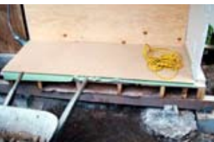
One area of the house torn apart to locate and eradicate the house fungus. Drastic measures were required, including cutting off floor joists.
