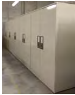
New steel cabinets in the basement of the Burke Museum.
